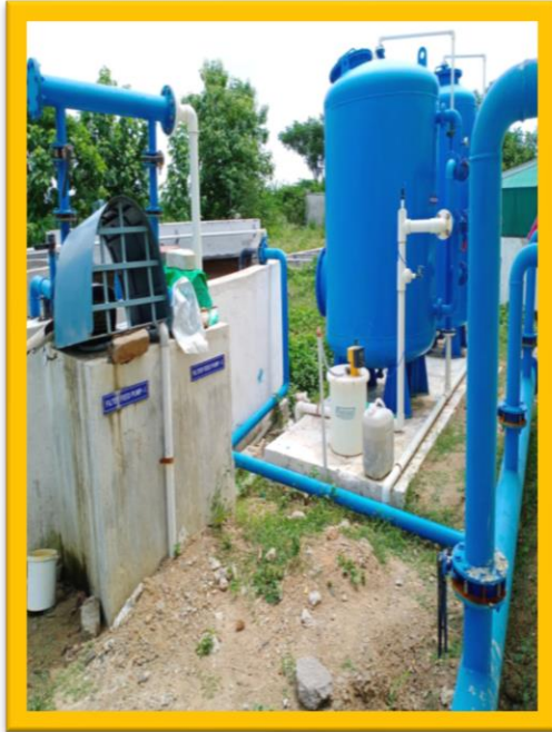
Filter Feed Pump – I & II
