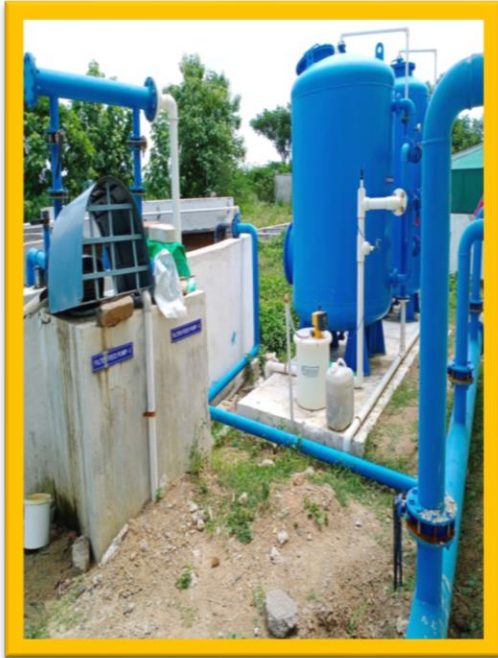
Filter Feed Pump – I & II
